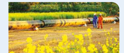
World's longest heated and insulated oil pipeline
