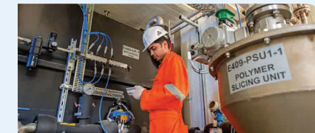
World's largest Enhanced Oil Recovery (EOR) polymer flood project
