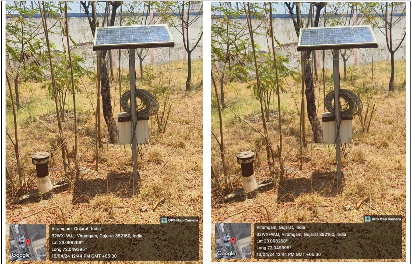
Viramgam terminal Piezometry fitted with telemetry
